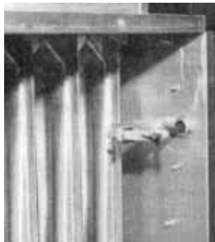
View of limit switch from "inside" the furnace
