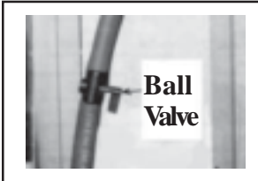
FIGURE 13 - Disconnect the power and adjust the water flow with the ball valve.
