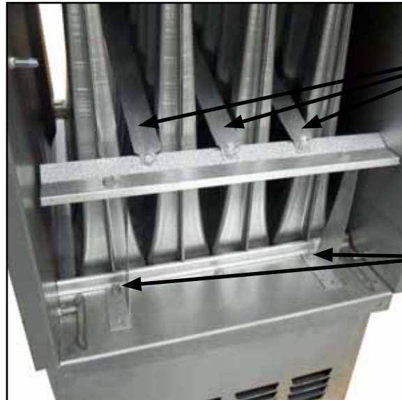
FIGURE 28 - Discharge Air End of the Heat Exchanger showing the Baffle Assembly to be Removed
